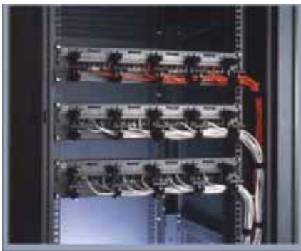
Netserver – rear cabling
